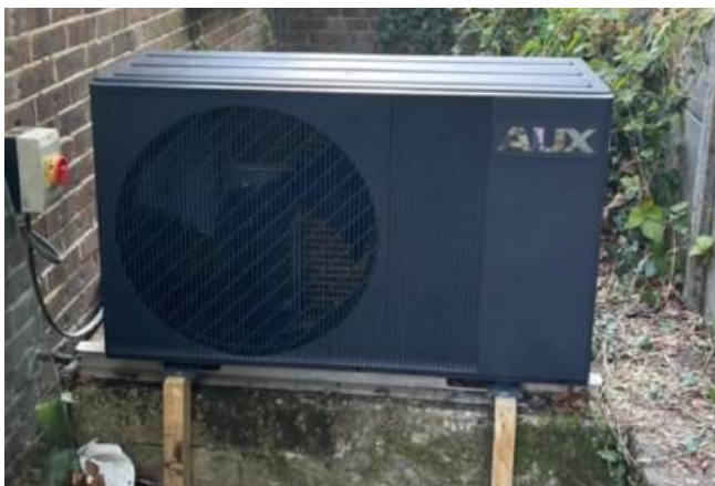
The newly installed outdoor Air Source Heat Pump unit
